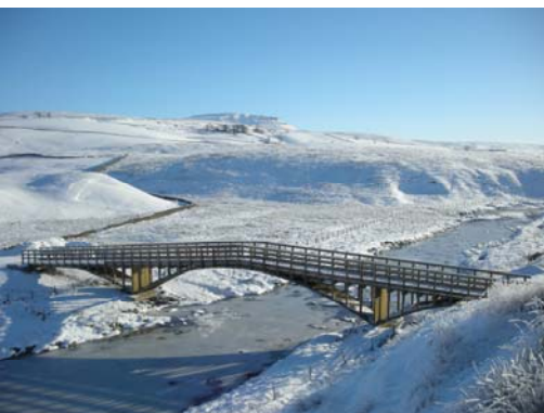
The award winning Farmoor Bridge, part of the newly opened Pennine Bridleway National Trail
